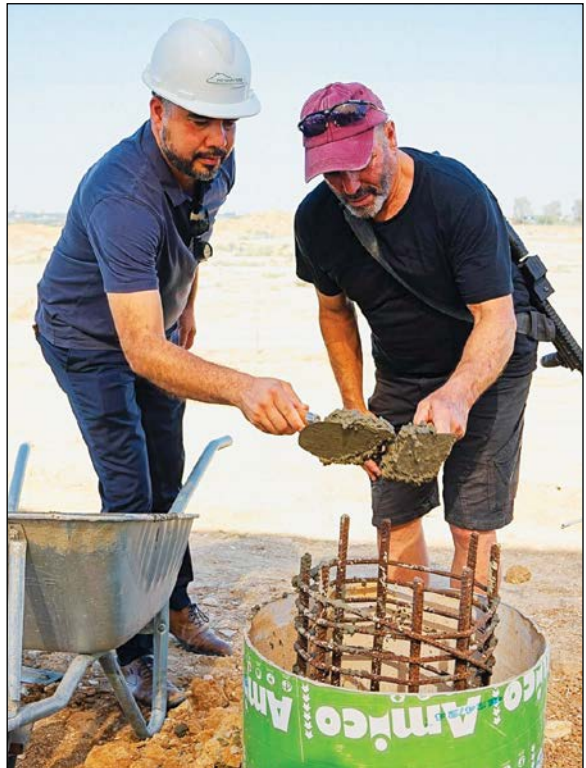
Bridges for Peace Israel Operations Director Daniel Kirchevel (left) helps lay the foundation stone for the new neighborhood in Kibbutz Be’eri alongside a community member.
